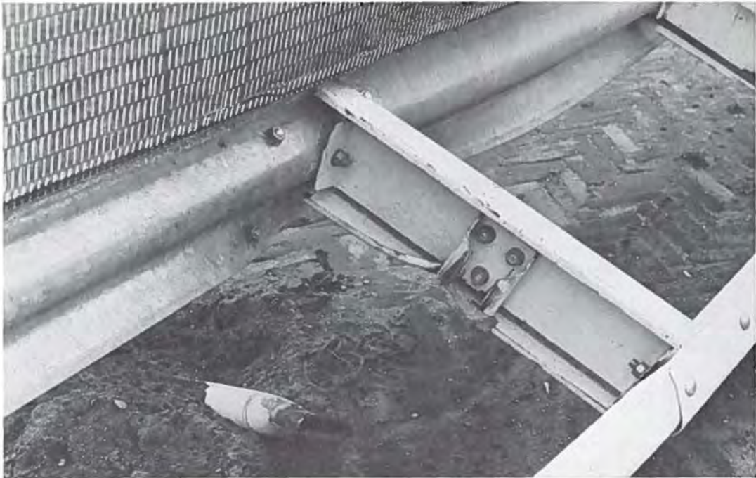
Figure 10. Post run over after breakage of rupture device.
