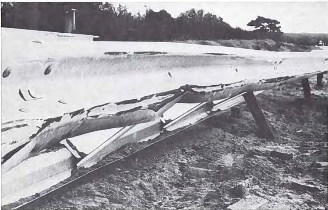
Figure 21. Denting of bottom flange in front rail with severe impact.
